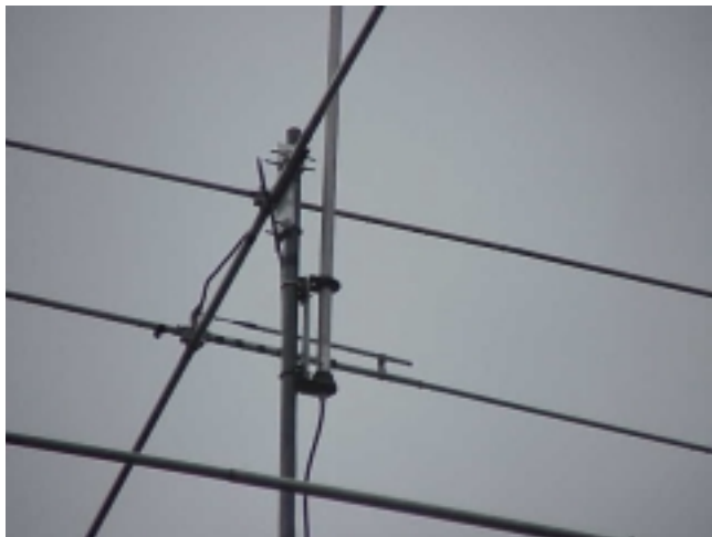
Close view of the mounting bracket for the antenna. The bracket is grounded to the mast but the antenna is insulated from the bracket.
